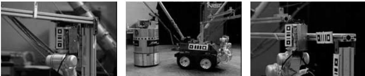
Figure 10 – Steps in the assembly process. Crane brings the beam close to the upright supports. The Mobile Manipulator grasps one end and docks it in one support. (“near end”, left) The Mobile Manipulator turns around, drives to the second support. (“swap ends”, middle) In this case, the Mobile Manipulator guides the beam in the horizontal direction while the Crane lowers the beam into place. (“far end”, right)
